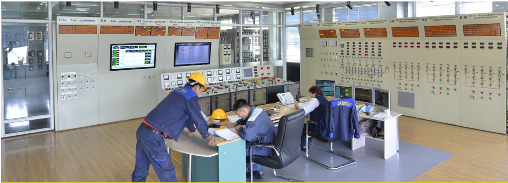
Control center of a power plant investment project in Ulaanbaatar, Mongolia.
